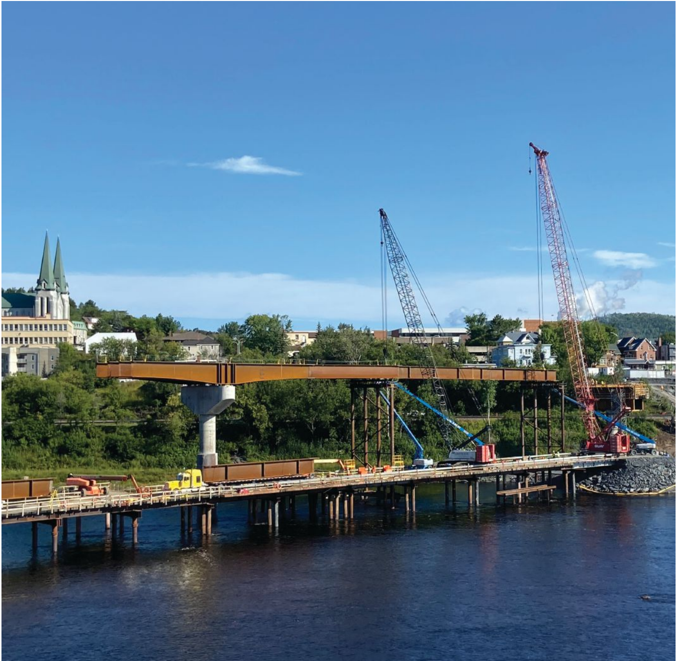
The I-shaped plate girders are made of Grade 50W and 70W uncoated weathering steel.
